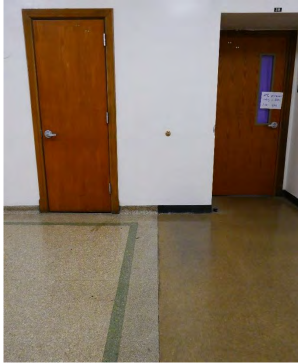
34 5/27/2022 Facing E Hallway floor material at connection of 1926 building (L) and 1963 classroom addition (R)
